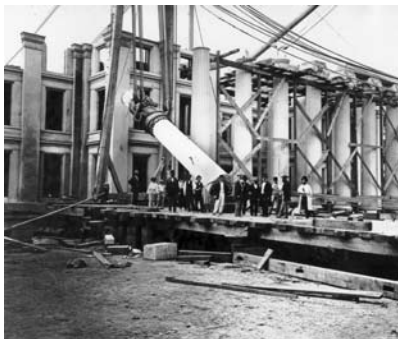
Solid granite columns are hoisted into place on the north portico of the Treasury Building, September 16, 1867. (National Archives)
